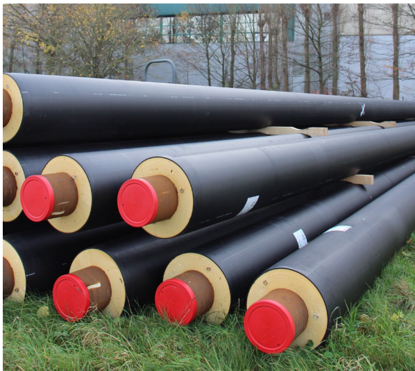
New District Heating installation at the IMOG WtE Plant, Belgium. © IMOG
