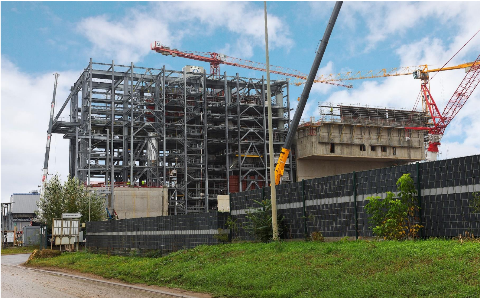
WtE plant in Wiesbaden, Germany, by courtesy of Doosan Lentjes GmbH.
